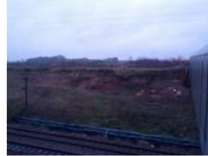
Perched Water table instability (Tills over Clays) Brantham Hall 2014
