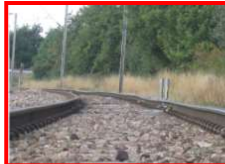
Clay Desiccation Track instability Great Bentley 2009
