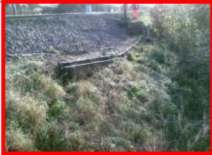
Deep seated London Clay embankment instability Chelmsford 2009
