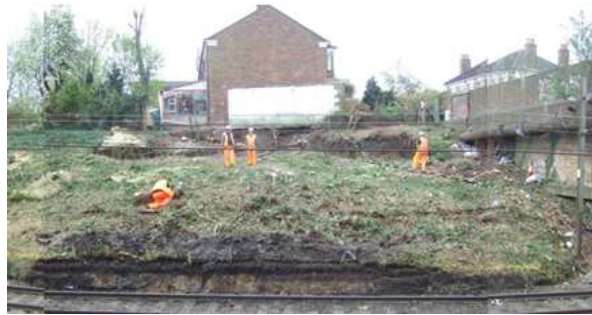
London Clay cutting slope failures Walthamstow Central 2009
