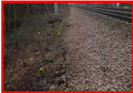
Ash degradation /instability Nags Head Lane 2016
