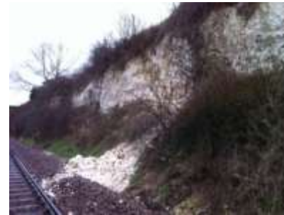
Chalk Slope instability Coalpit Cutting 2013
