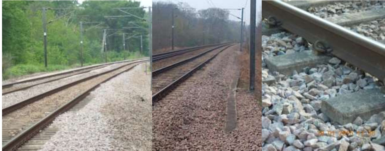
Sleeper Ends Exposed - Twist Fault
